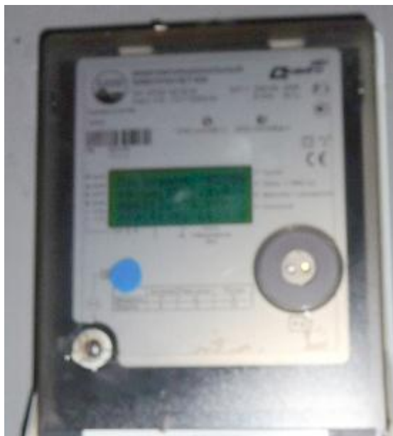
Figure 1 Electricity meter EPQS
