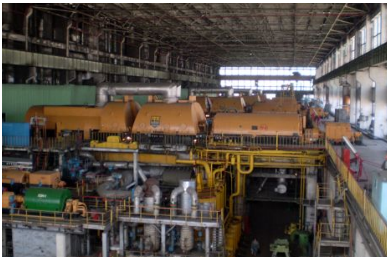
Figure 1. The Turbine Hall of the Zaporizka TPP.
