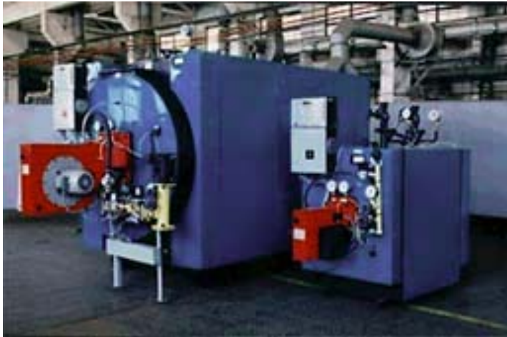
Fig. 3. Boiler VK-21 with efficiency 92%.
