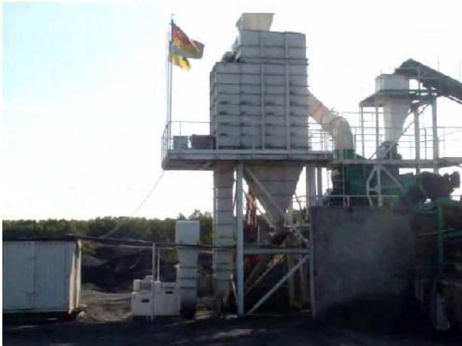
Fig.1 Project activity equipment
