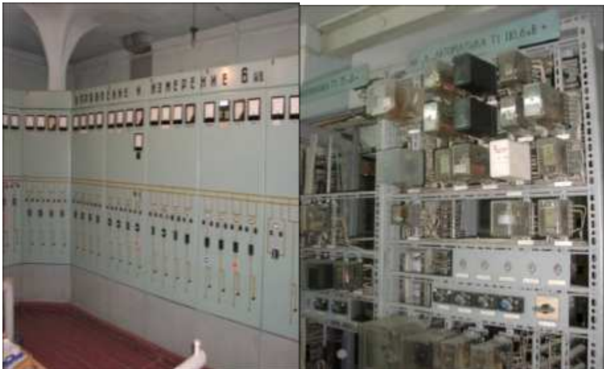
Figure 6. The Control Panel of the Substation before and after the Reconstruction
