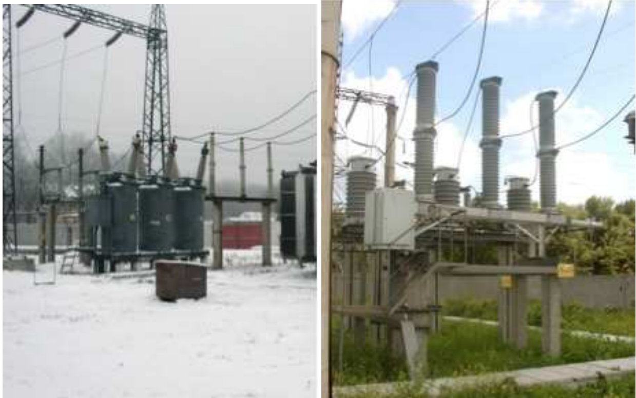
Figure 5. The Circuit Breakers before and after the Reconstruction.
