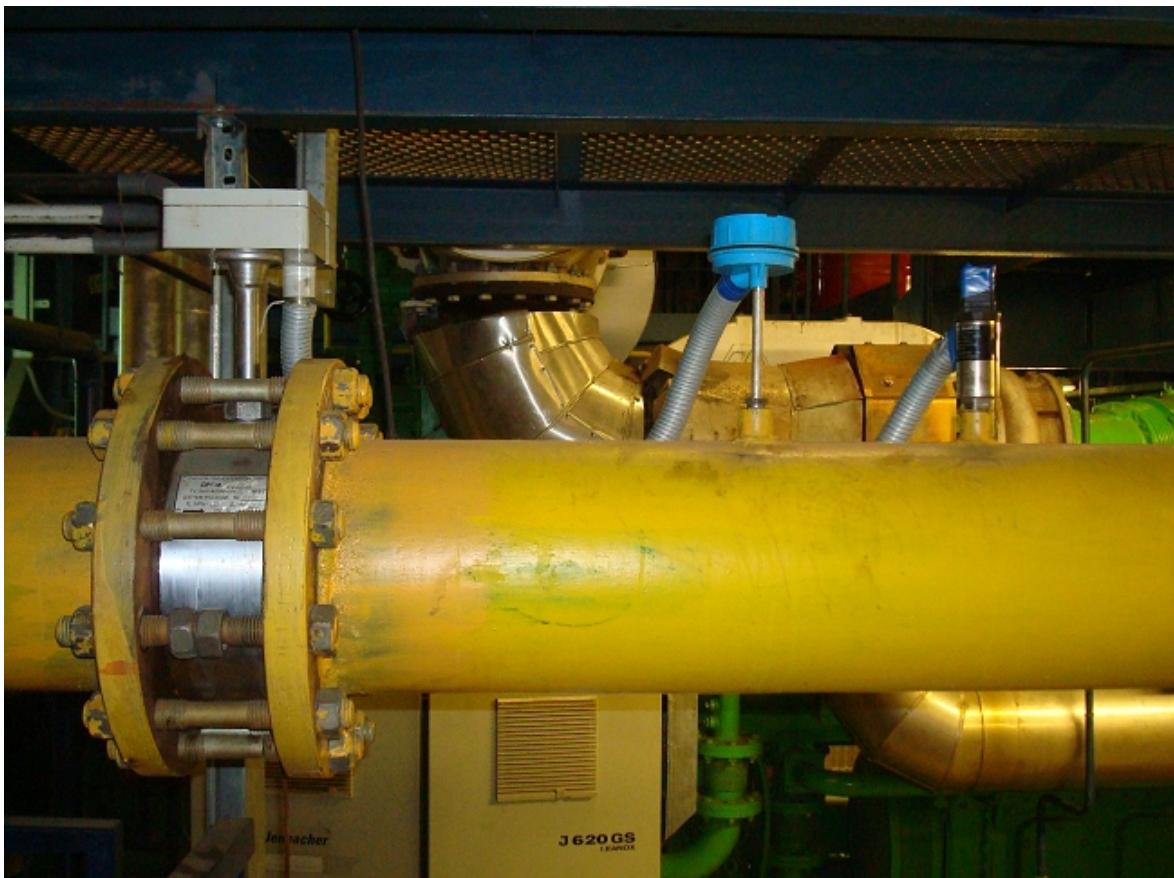
Figure 5: Gas flow meter DRG.M-10000 12 temperature sensor Metran 274-02 and pressure sensor Vegabar-14 of metering system for gas record BKT.M at fuel gas pipeline of SU CHP unit.
