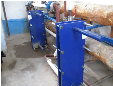
Fig. 1 New heat exchangers
