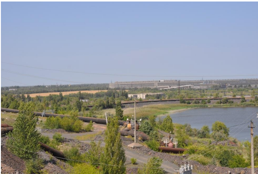
Figure 2 Gravity service water supply pipelines at PJSC “InGOK”
